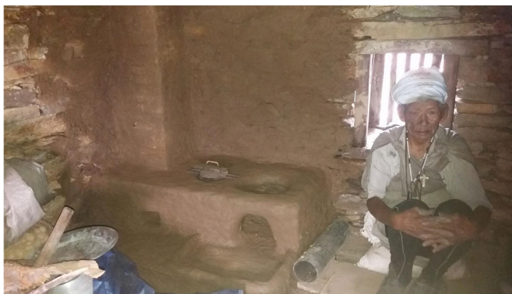
Proud owner and newly built clay stove, metal pieces fitting, drying and firing to be done
